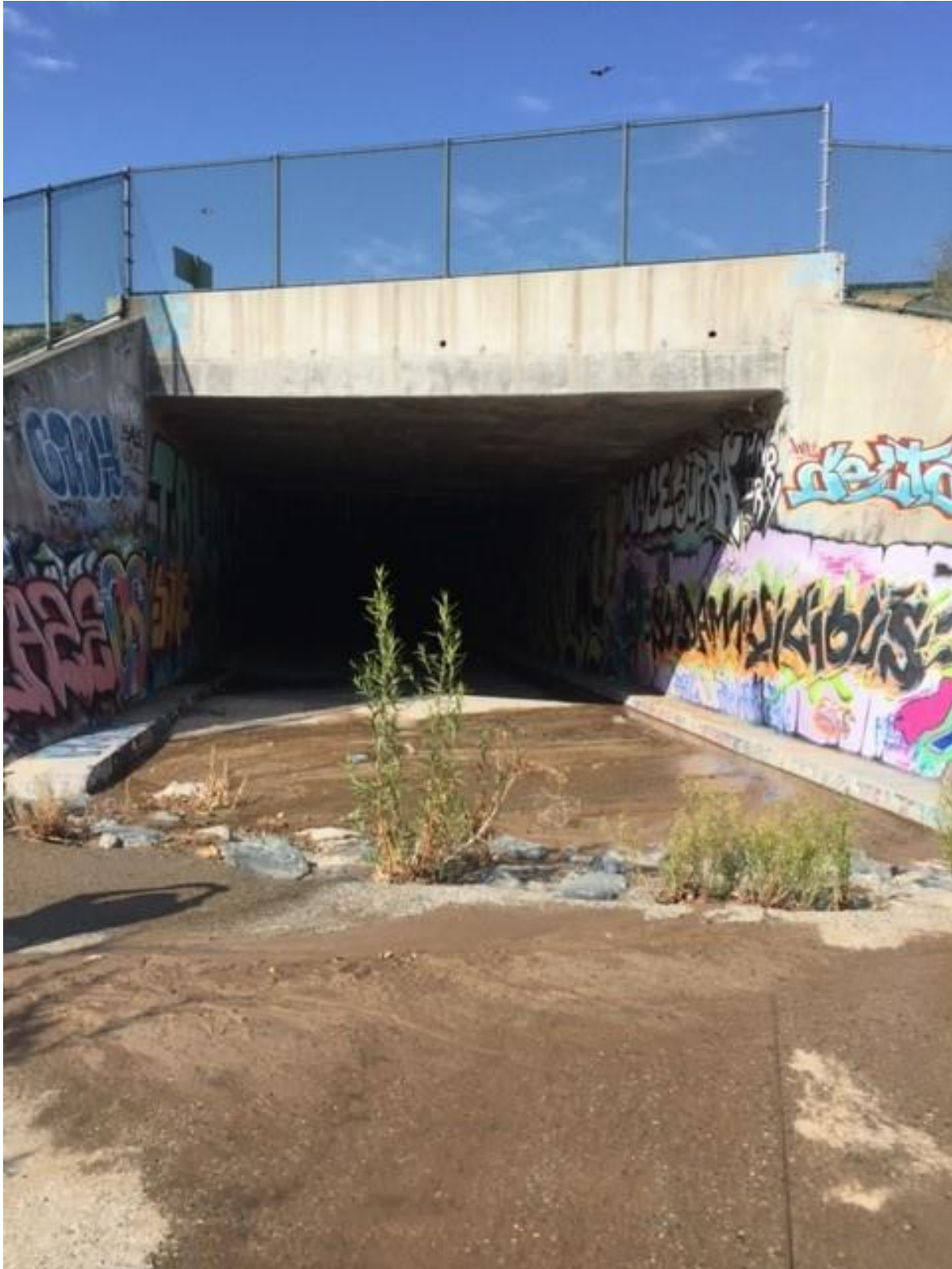
Figure 4. The I-5/I-405 interchange underpass shows extensive human usage.
